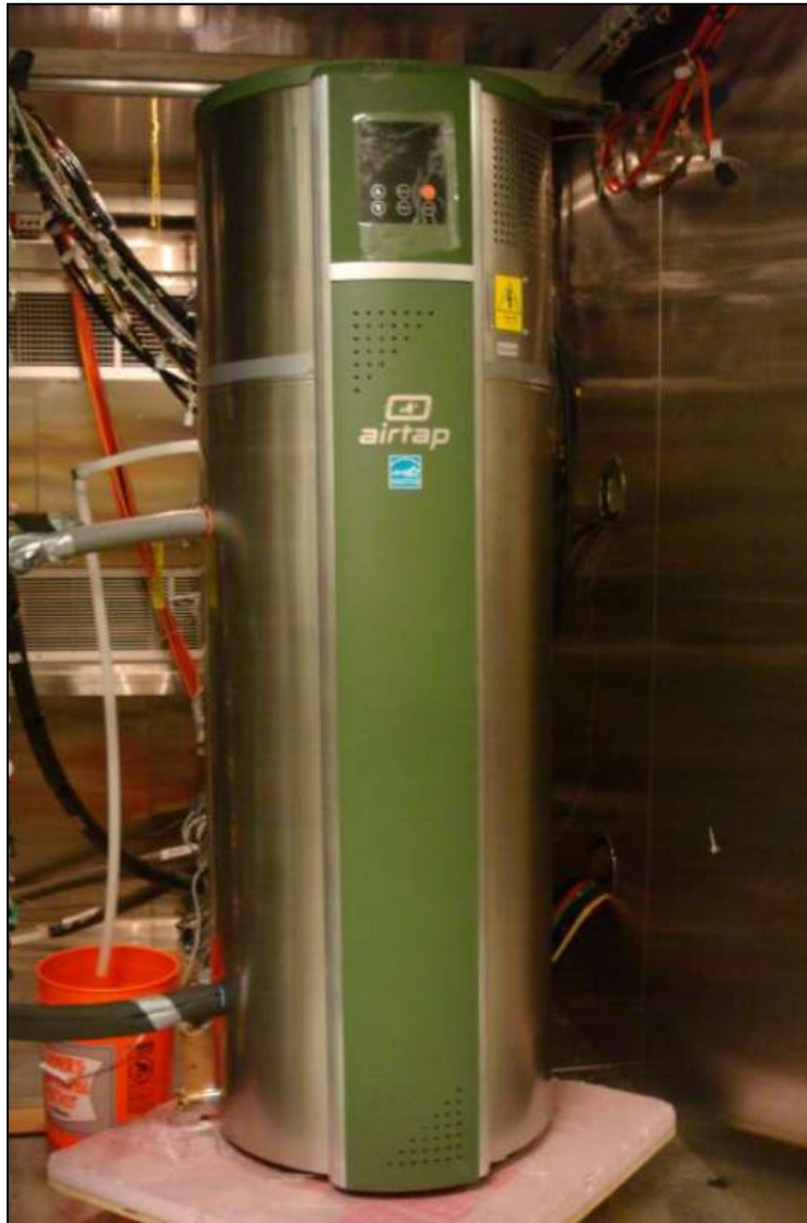
Figure 1. HPWH Test Unit Installed Inside Thermal Chamber
