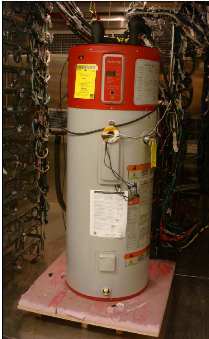
Figure 1. HPWH Test Unit Installed Inside Thermal Chamber
