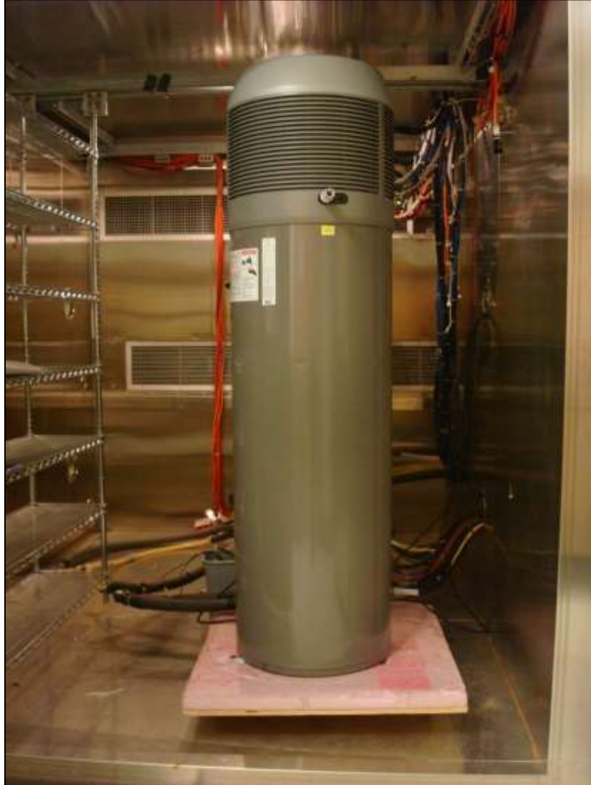
Figure 1. HPWH Test Unit Installed Inside Thermal Chamber
