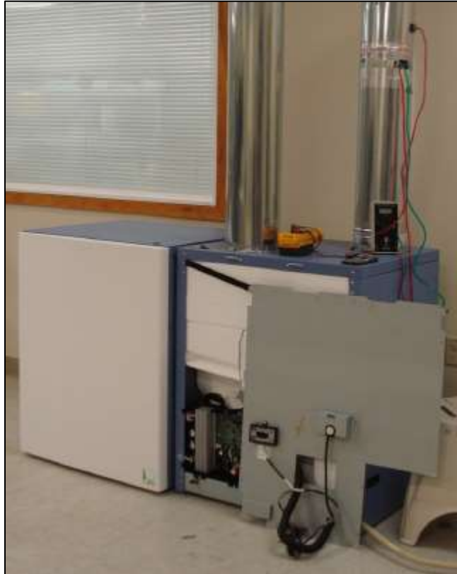
Figure 6. Fan Test Setup and Duct Connections
