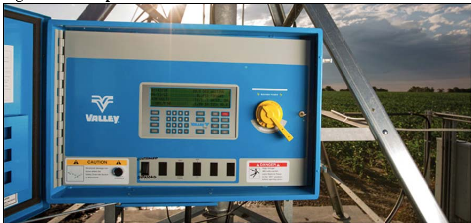
Figure 10. Example of Pivot Control Panel
