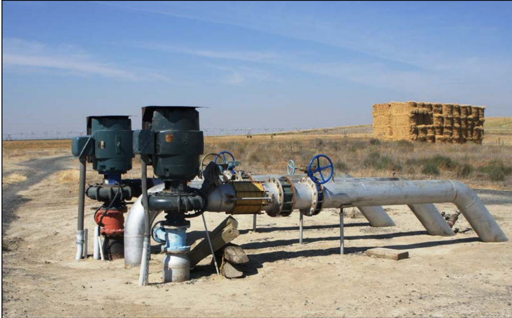
Figure 16. Pumps Feeding Water to a Center Pivot
