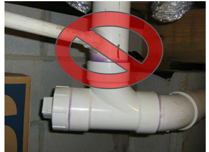
Can't tie into waste line
