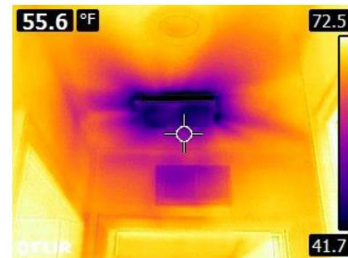
Thermal image with Blower Door – air leakage at whole house fan
