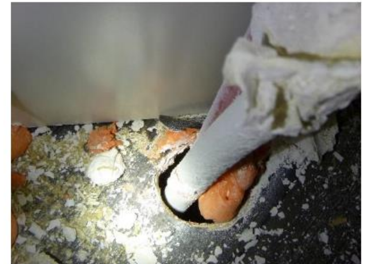
Broken plumbing penetration seals under sinks
