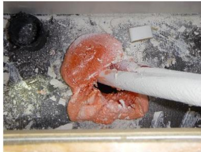
Broken plumbing penetration seals under sinks
