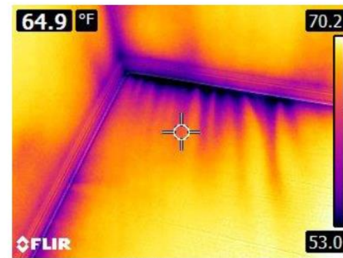
Thermal image with Blower Door – air leakage at bottom plate of wall
