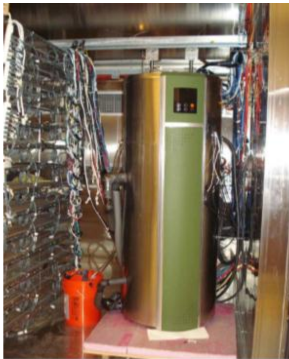
Figure 1. HPWH Test Unit Installed Inside Thermal Chamber
