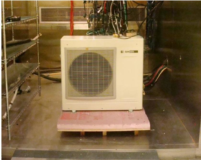
Figure 1. HPWH Outdoor Unit Installed Inside Thermal Chamber
