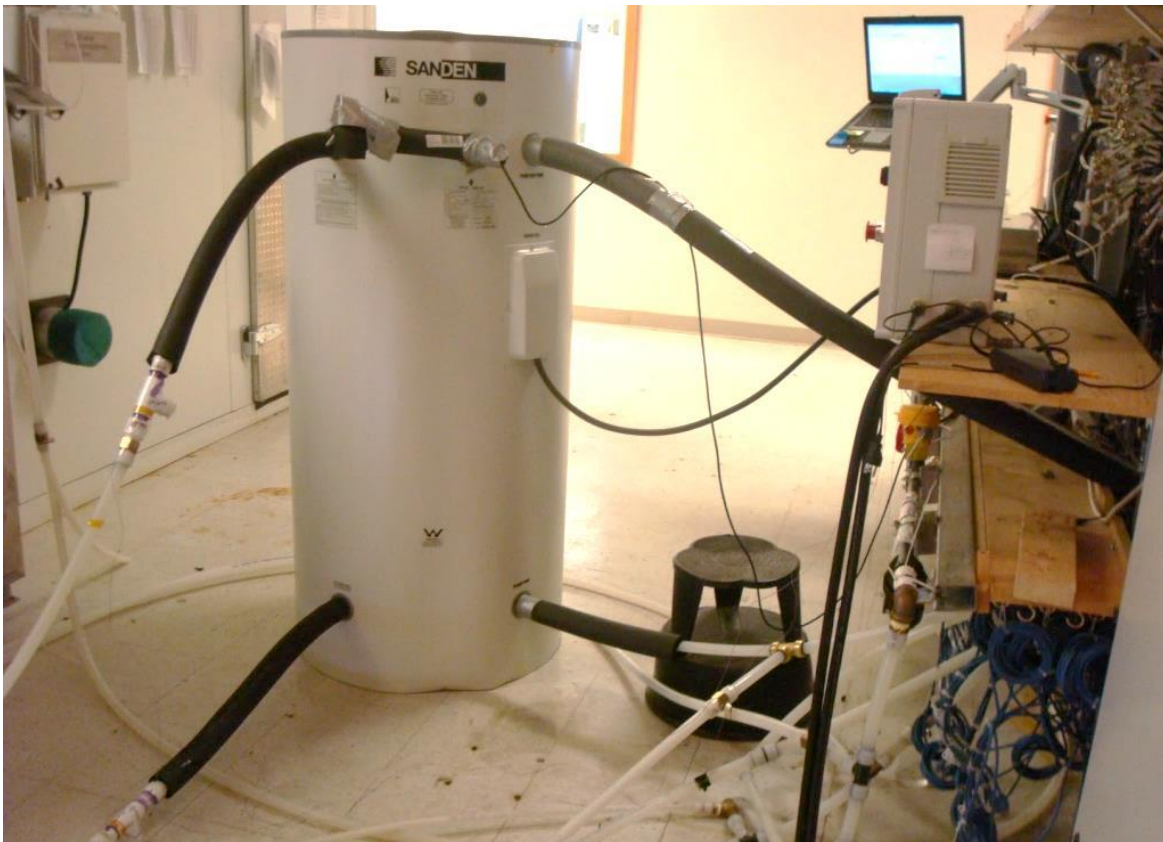
Figure 2. Hot Water Tank Instrumented and Installed Adjacent to Thermal Chamber
