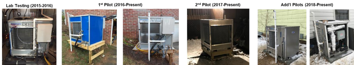
Figure 6: Photos of Low-Cost GAHPs Operating in Prior/Concurrent Residential Heating Demonstrations
