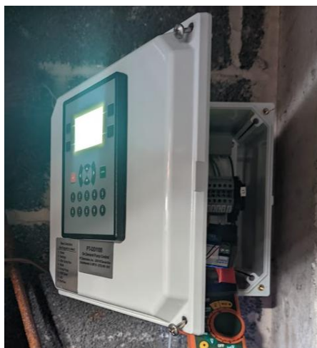
Figure 63: DHW On-Demand Recirculation Pump and Controls
