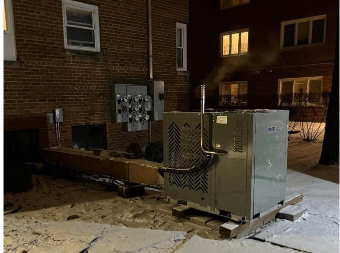
Figure 1: GAHP Unit Installed at Evanston, IL Multifamily Site
