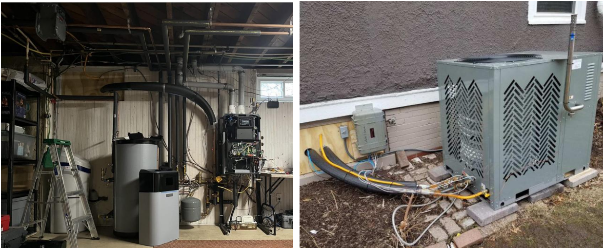
Figure 25: Single family GAHP Combi at La Porte Hydronic Heating Site
