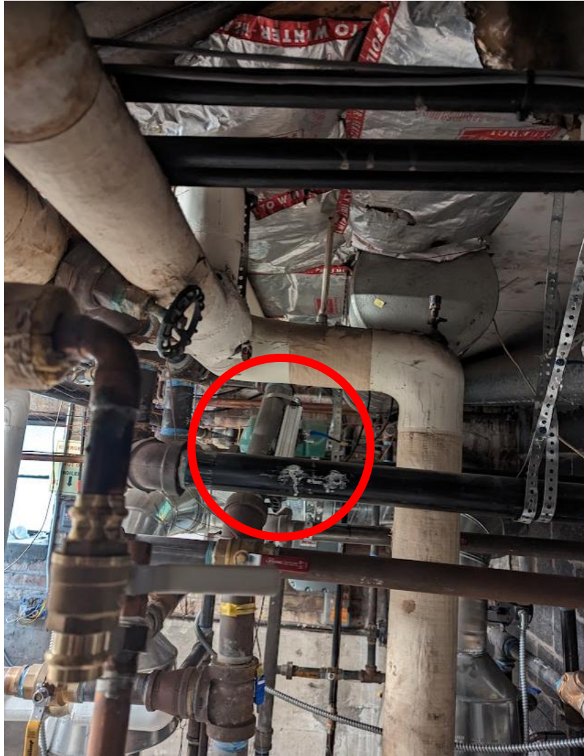
Figure 65: Relocation of Ultrasonic Flow Meter to Main System Space Heat Return to Zones on 3/6/2023
