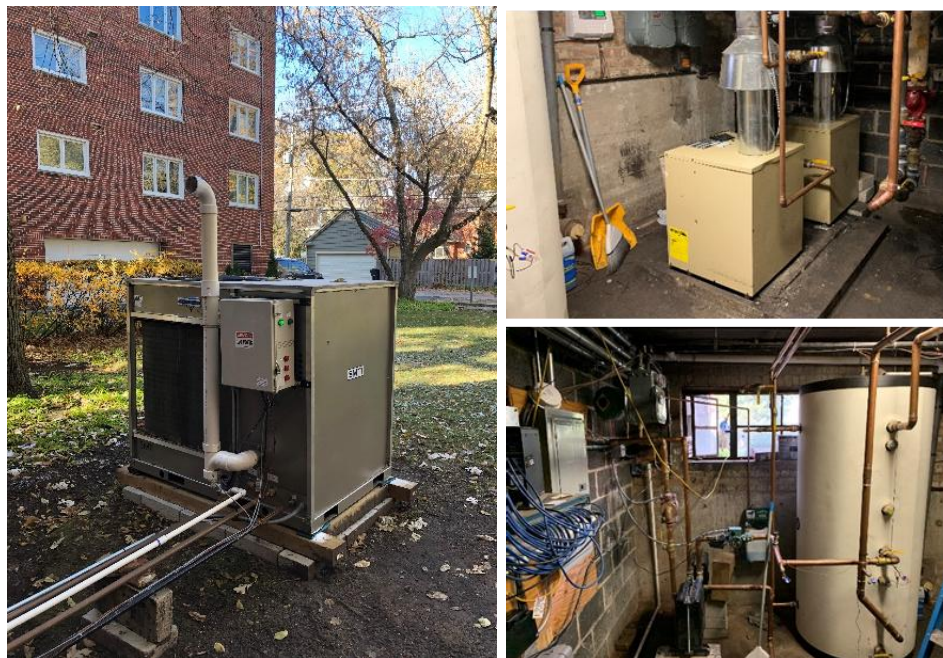
Figure 11: Multifamily Unit Site during Initial GAHP Monitoring Phases (2019-2021)
