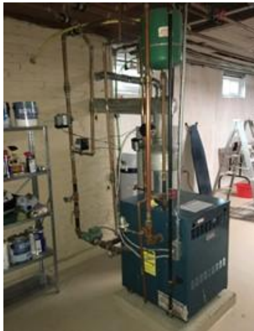
Figure 13: Original Boiler and Water Heater at La Porte Site
