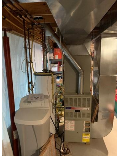
Figure 17: Original Boiler and Water Heater at New Carlisle Site
