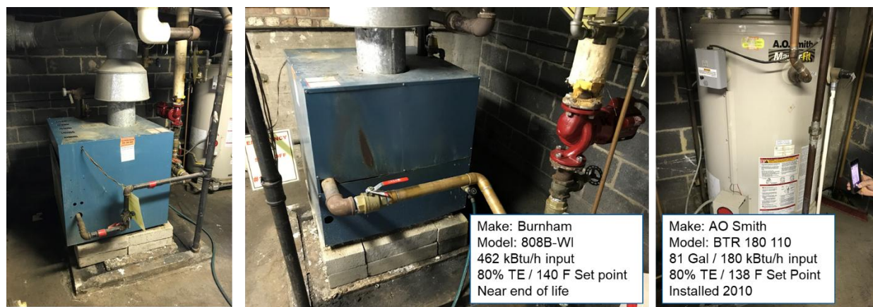
Figure 7: Original Boiler and Water Heater at the Multifamily Demonstration Site
