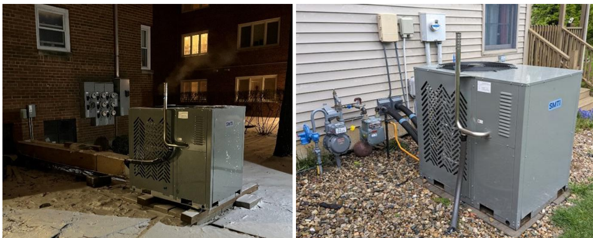
Figure: Multifamily (Left) and Single Family GAHP Installations for this Demonstration
