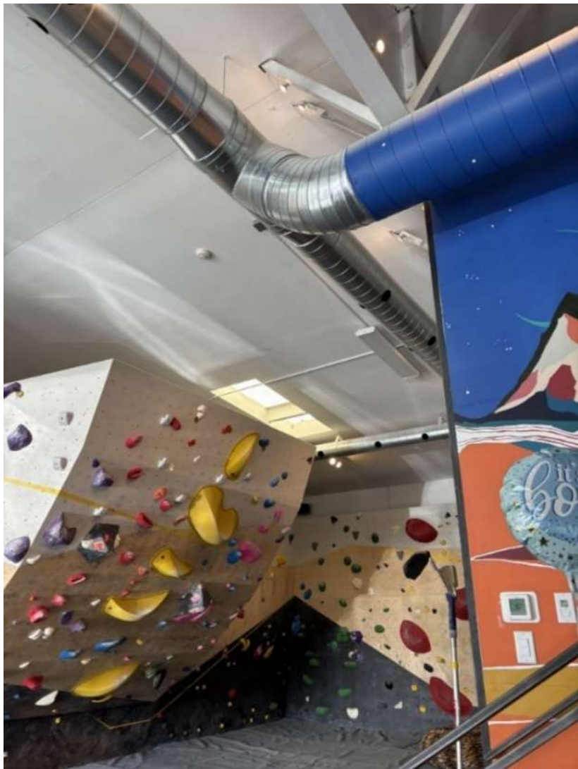
Figure 2 - Newly added climbing wall area, serviced by an HRV.
