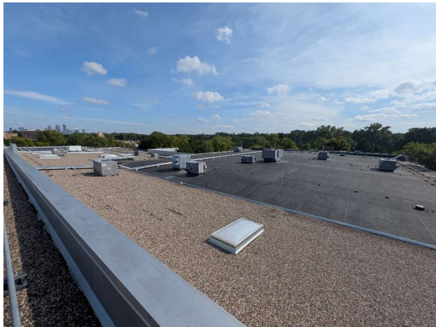
Figure 4 - RTU ERV (and other HVAC) atop an office complex.
