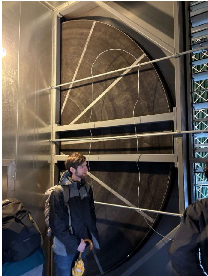
Figure 3 - Example of a very large rooftop, wheel-based HRV.
