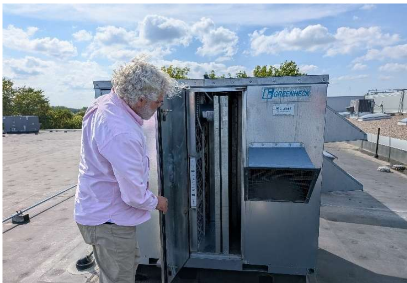
Figure 1 – Roof Top Unit (RTU) wheel-based ERV at a furniture design center.
