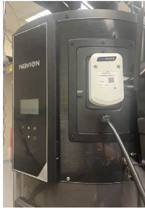
Figure 20: CTA-2045 Module installed on the DF-HPWH.
