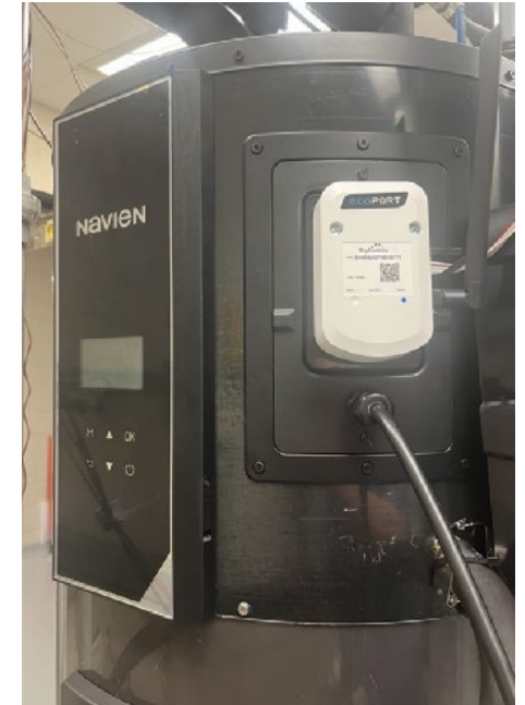
CTA-2045 Module installed on the DF-HPWH.
